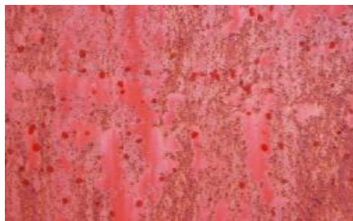
Obr. 10 Detail koroze plechu
