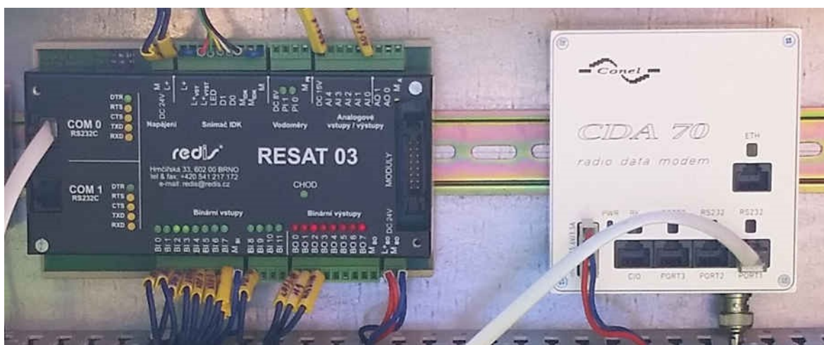
Obr. 3.10 PLC Resat03 a radiomodem CDA70 [10]
