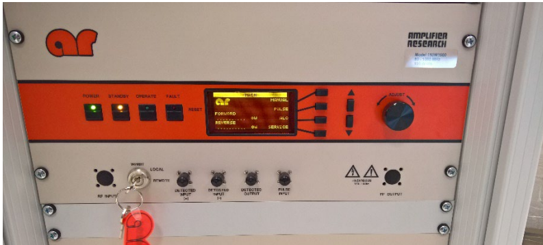
Figure 41. 150 W RF power amplifier
